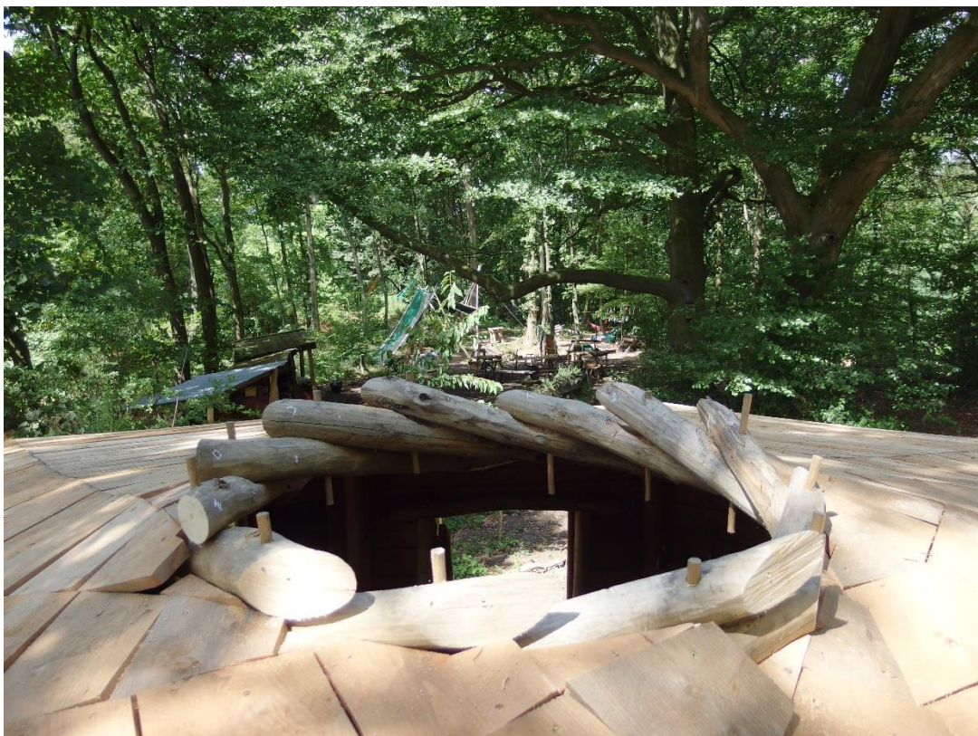
4 th August 2018 - cutting the ends of the roof poles, ready for felting
