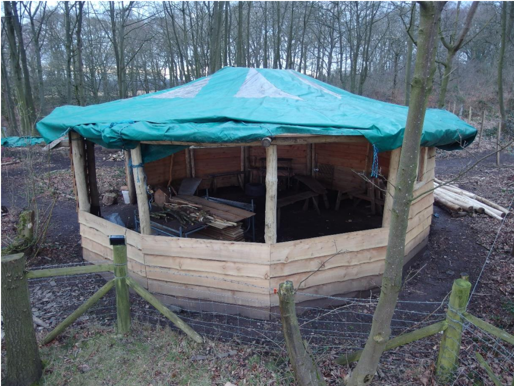
4 th February 2018 - first layer of roof complete and covered by waterproof tarpaulin
