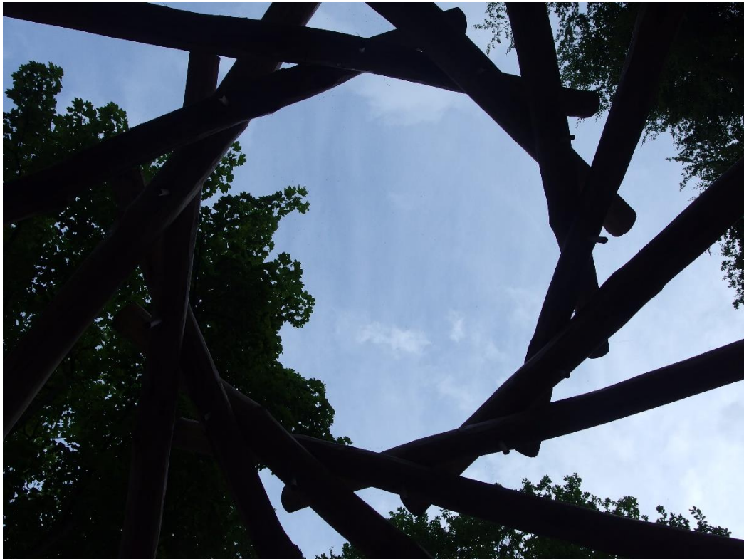
8 th July 2017 - view through the roof, now in place and secured with more oak pegs!
