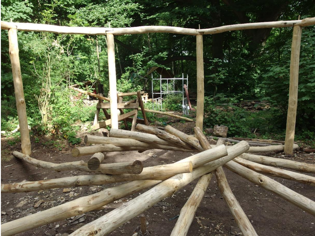
7 th July 2019 - detail on reciprocal roof joints, showing how sculpted poles locate with each other
