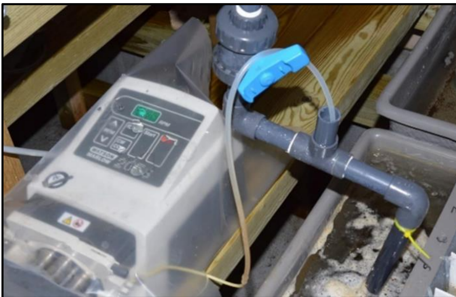
Figure 1. Picture showing one of the peristaltic pumps (Watson Marlow 205S) delivering chemicals to the operating water through a silicon tube inserted into an extension pipe on top of a mixing pipe leading the test medium into the experimental channel.
