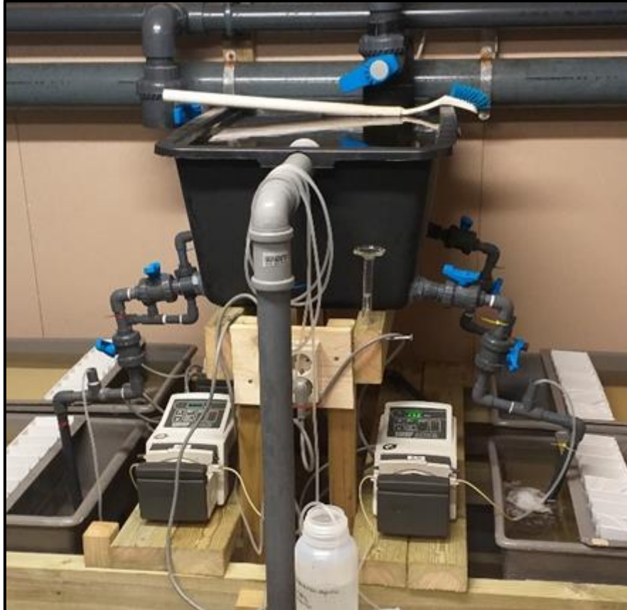
Figure 3. Picture showing the level tank (black tank). The large pipe in front of the tank is the overflow, draining the excess water ensuring a stable water level in the tank. The four smaller pipes on the tank sides are the mixing pipes leading water from the tank to the experimental channels. Over the tank, in the background, is the inlet to the level tank supplying it with the operating water (large blue lever).
